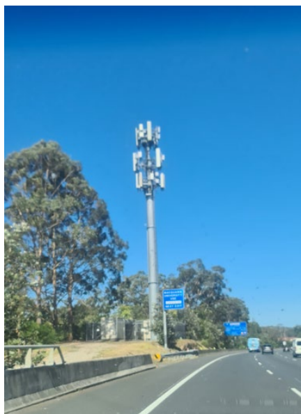
Image 2: Example of a monopole tower with the 3 mobile network operators co-located on the tower.
